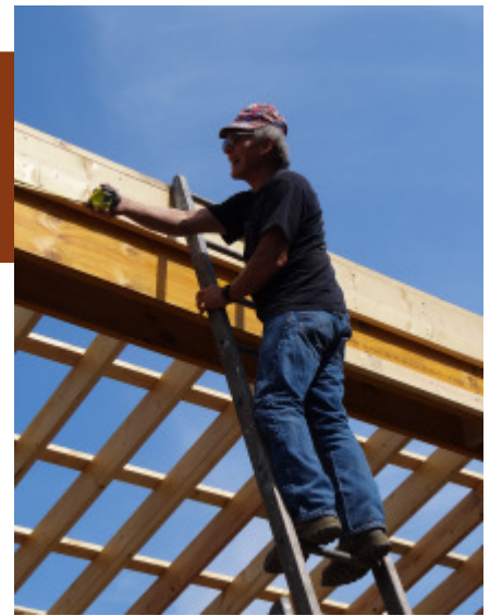
(Above) Bentley Hudson, retired commercial electrician, has no fear of heights as he measures the top of the building.
