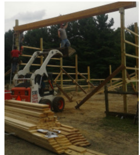
(Above) Walter Shields balances in the bucket of the skidsteer as the front boards of the top of the building are put into place.
