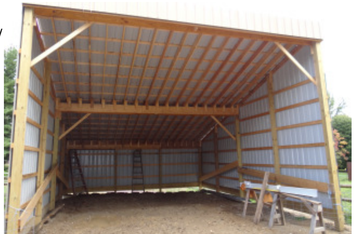
(Above) Before the concrete is poured. We'll provide everyone with a photo of the completely finished building in the next newsletter.
