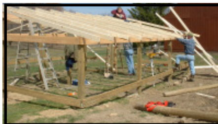
Russ Fisher (on roof) and Dick Zampini (right) level boards for the roof of the barn.
